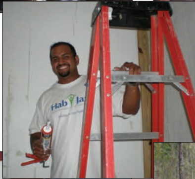
Suneil Kutbiala, joined others from CSX to help caulk and paint the Seamark commissary.
